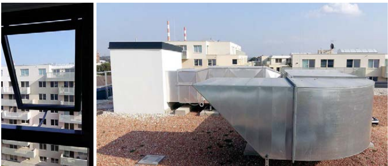
Figure 2. Air inlet window with chain actuator (left) Exhaust ventilator on roof (right).
