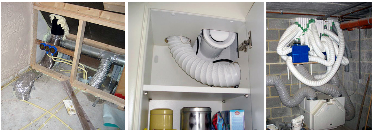
Figure 6. Installations of residential ventilation systems.
