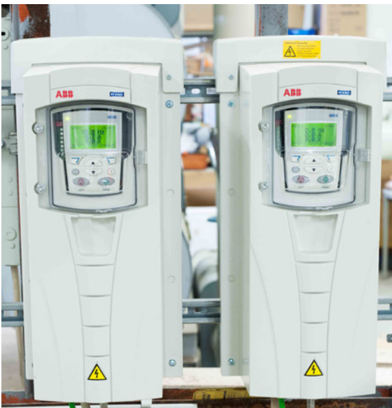
Figure 5. Two HVAC ACH550 drives regulate the pumping of the substation.
