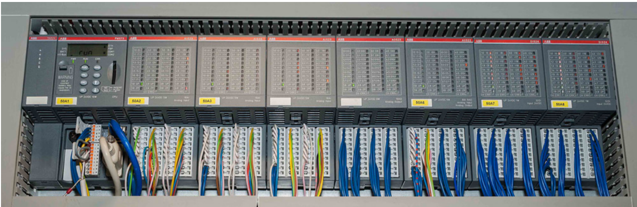
Figure 4. The PLC in the pipe cellar regulates six heating circuits of a large and complex ventilation system.
