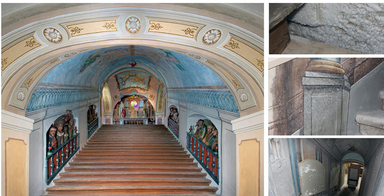
Figure 1. The Pilgrimage chapel of Holy stairs [10]. Frost on the frescoes leading to damages.
