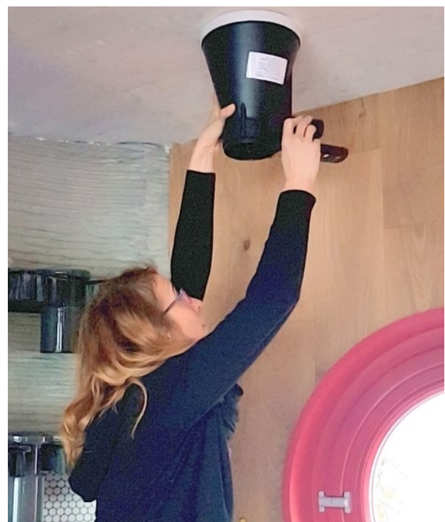
Figure 4. Verification of air flow at the exhaust of ventilation system.
