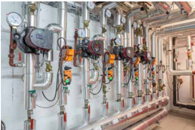
Heating distributor in the heating station.
