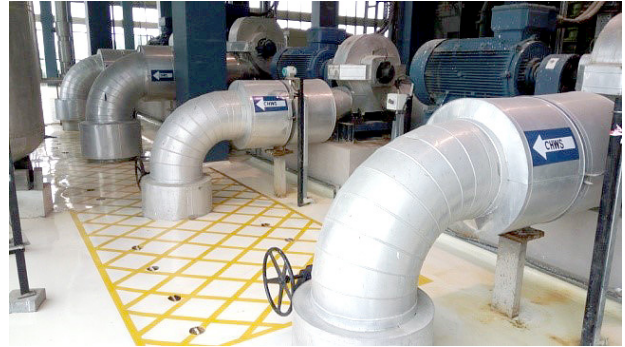
Figure 9. Chilled water pipe routed below the ground trench.
