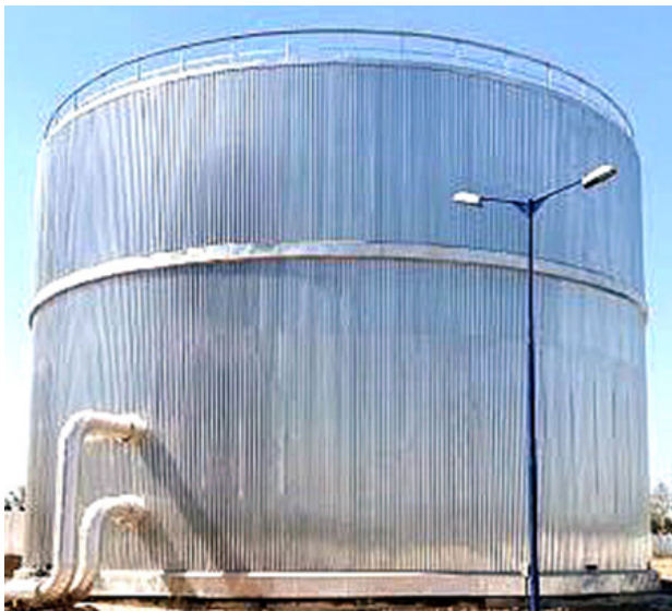
Figure 8. TES tank at DCP-1.
