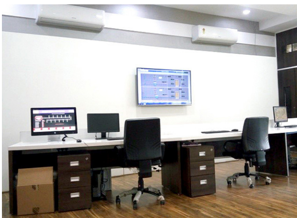
Figure 15. SCADA control room at DCP-1.
