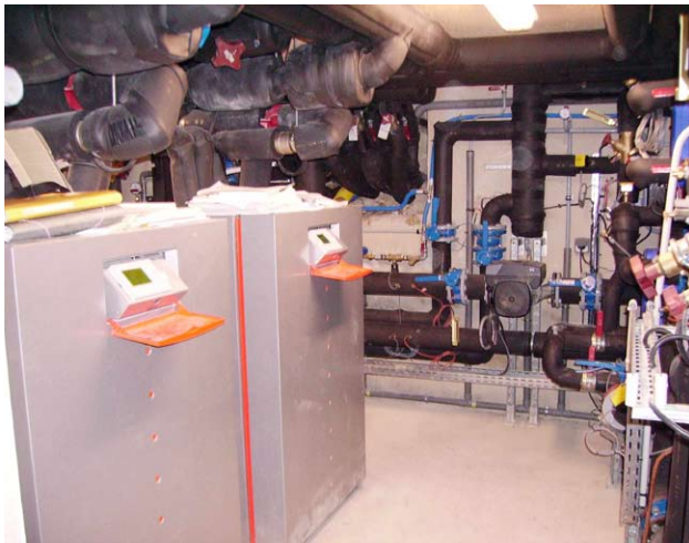
Figure 4. Water/water heat pumps.
