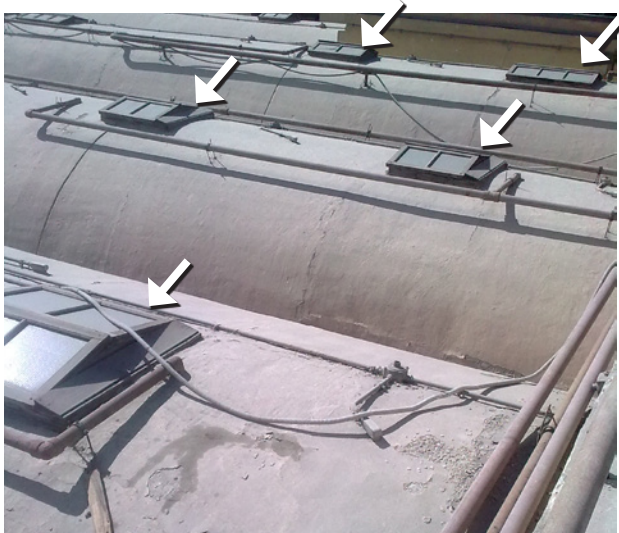
Figure 4b. Arrows indicate location of air inlets through naturally openings in the roof.
