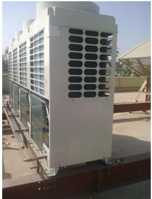
Figure 3. Cooling Equipment on Roof of adjoining building.
