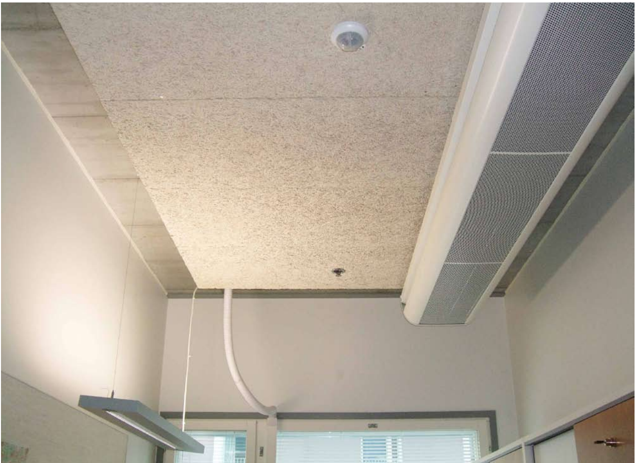
Active chilled beams and lighting fittings in offices.
