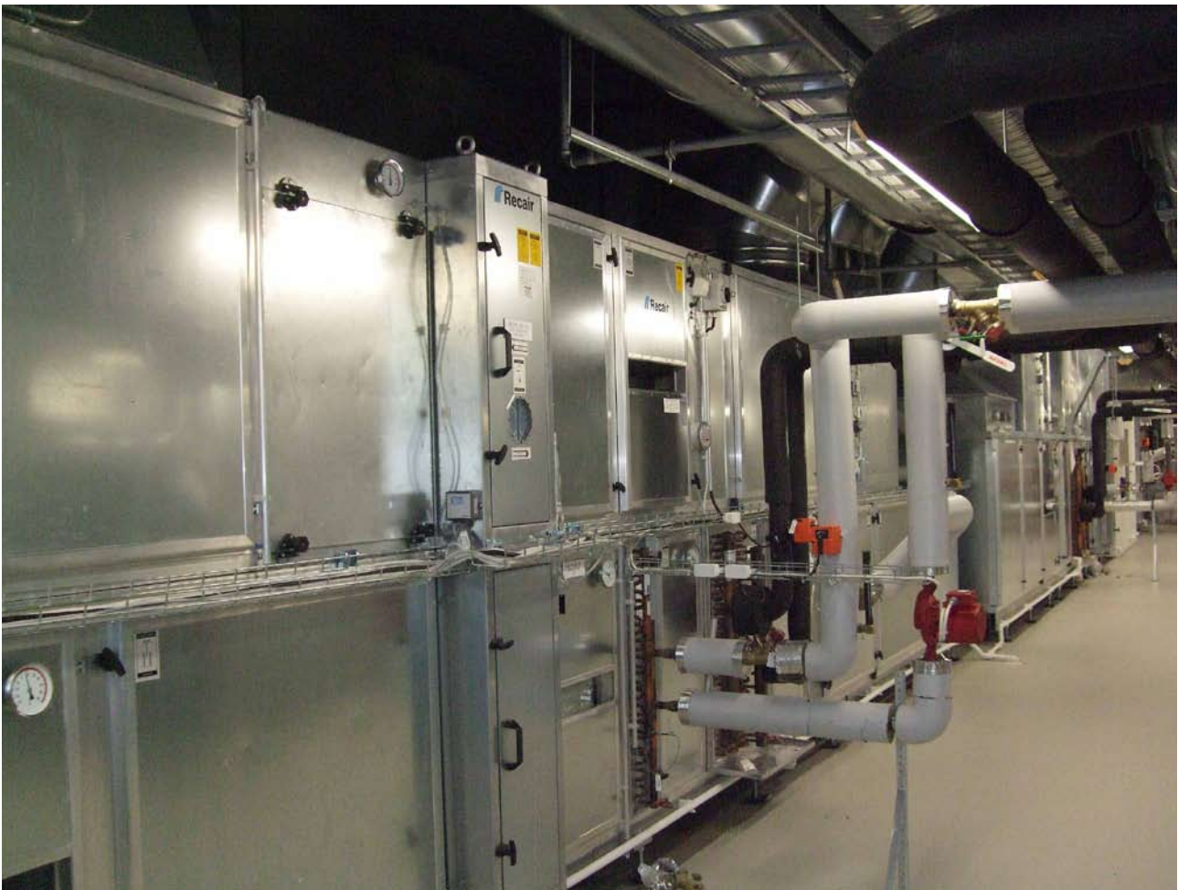
Large air handling units and ductworks have been used to achieve as low specific fan power as 1.4–1.6 kW/(m 3 /s) for offices and similar spaces and 1.8 kW/(m 3 /s) for VAV air handling unit serving meeting rooms.
