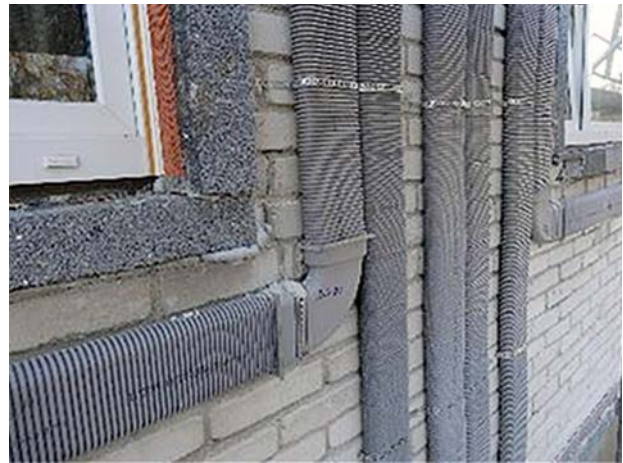
Figure 2. Supply ventilation ducts in additional insulation of external wall.
