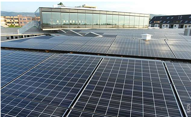
PV panels installed on the roof.
