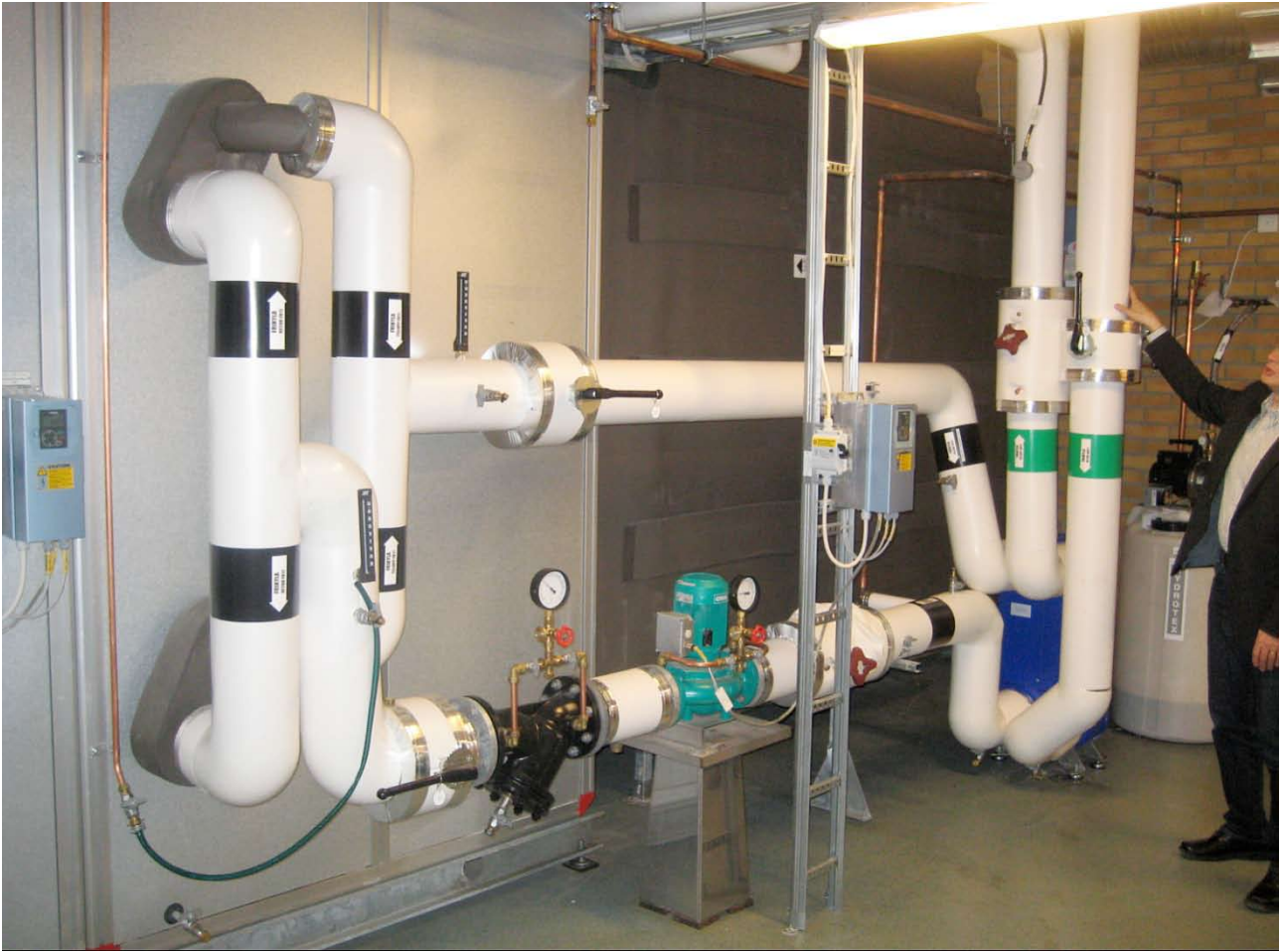
Figure 3. Free cooling coil as first step in the AHU. From the right: the heat exchanger that exchanges the heat from the glycol circuit in the coil in the AHU to the chilled water circuit for cooling beam system. Energy saving is approx 5 – 10 kWh/m 2 annually.
