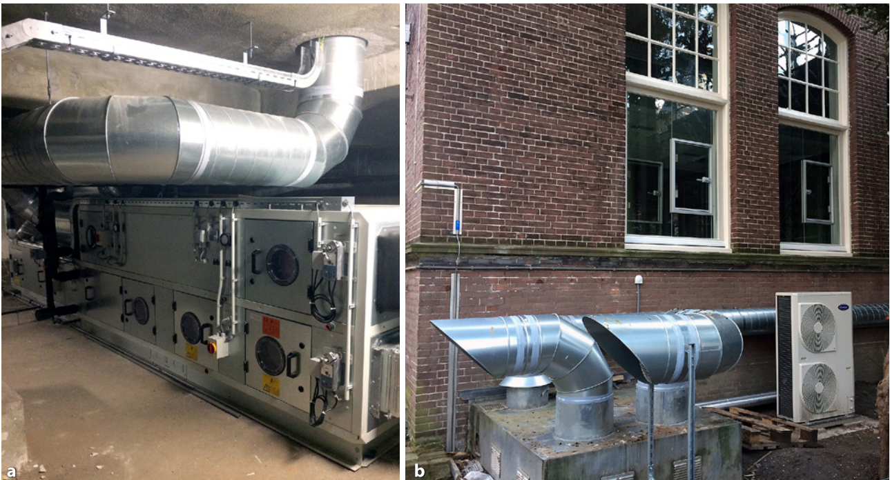
Figure 2. a) Installations in basement and b) cooling unit outside the SenseLab.
