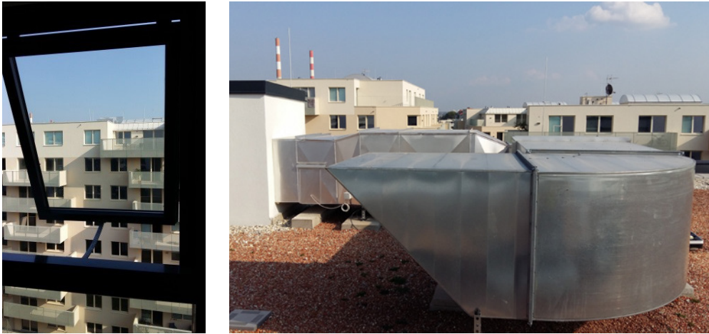
Figure 1. Air inlet window with chain actuator (left) Exhaust ventilator on roof (right).
