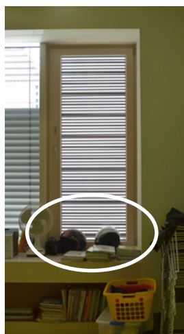
Figure 7. Window for manual night ventilation secured against rain burglary and fall but blocked by books.
