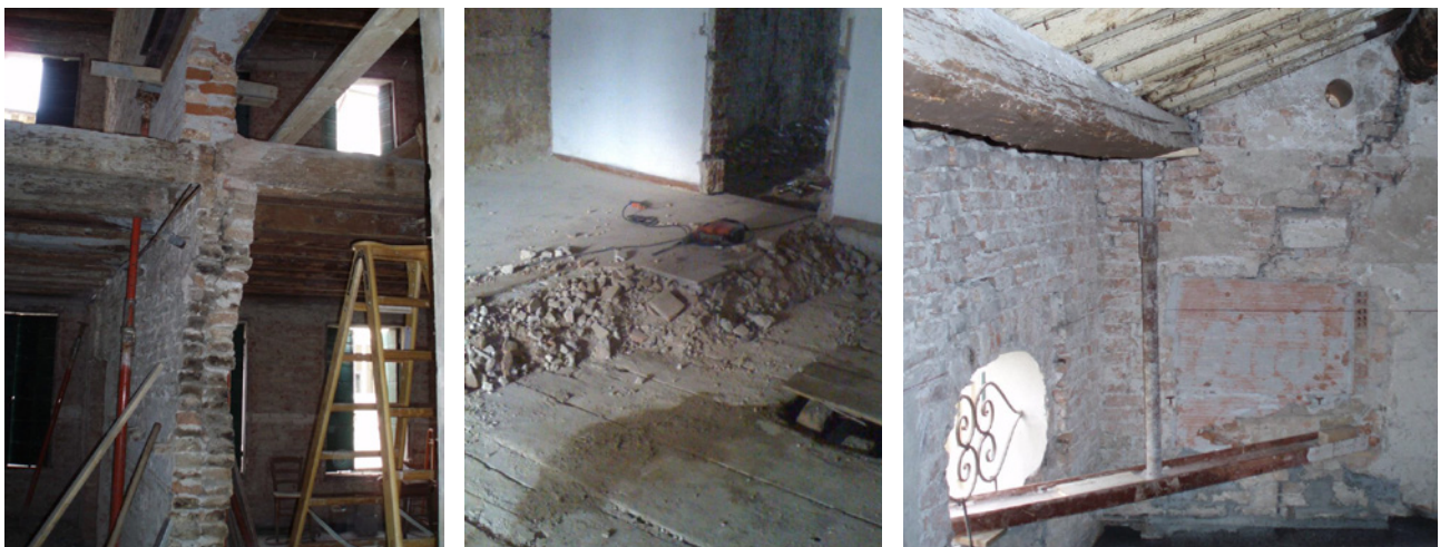
Figure 2. Building envelope before renovation: crooked walls (left), demolished partition walls left and used as a substrate (center), beam support in the perimeter wall (right).
