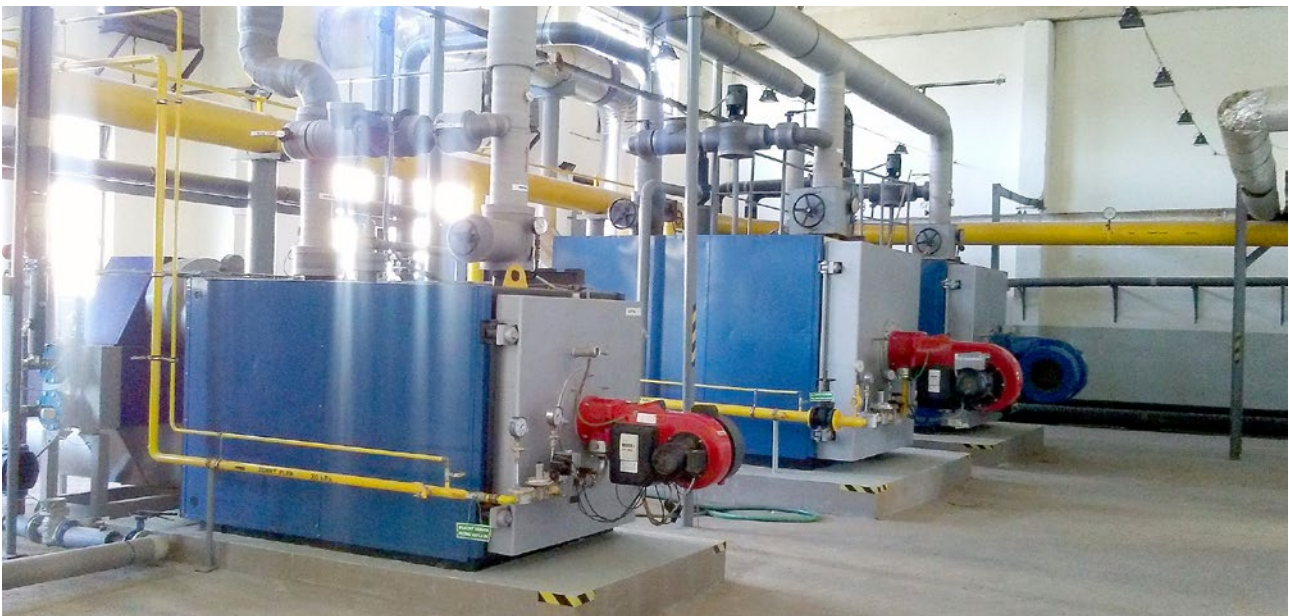
Figure 1. Interior view of the existing three hot water boilers [1]
