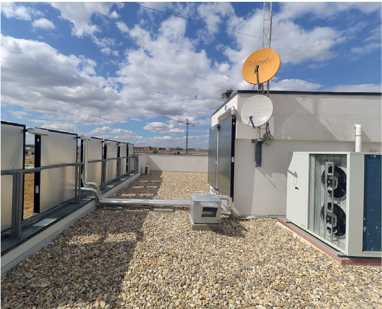
Figure 3. Heat pump and solar thermal field installation on the south facing parapet.
