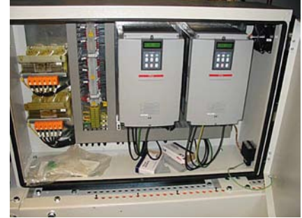
Figure 7. Electrical board with inverters for pumps.
