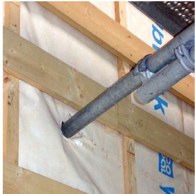
Figure 2b. Leaky wind barrier detail, from anchoring of the outside scaffolding (Photos: Tormod Aurlien).
