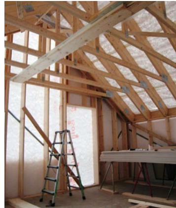
Figure 4. Norwegian wooden building being in early-wind-tight-stage. Wind-break layers are of nonwoven HDPE fabric. Some parts of the wall have gypsum boards in addition, to reach fire resistance goals.
