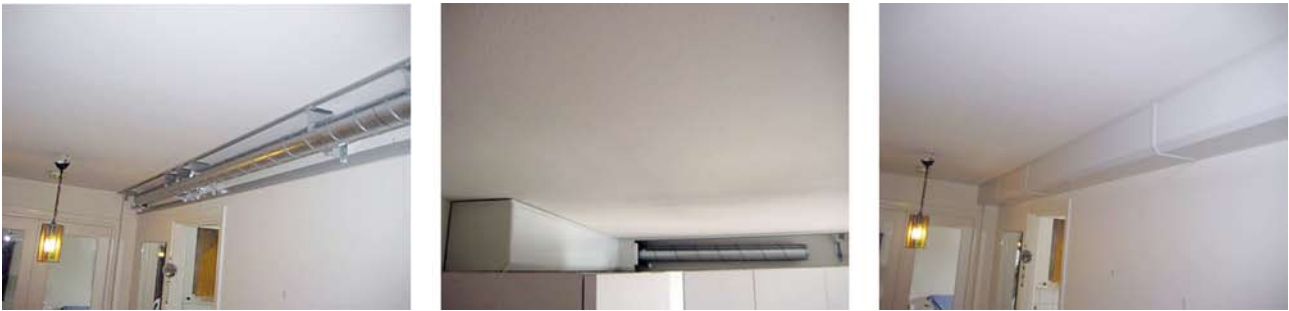
Figure 5. The supply air duct for the flat is fixed to a light framework at the ceiling. The duct is hidden behind a cladding fixed to the same framework – everything is done, quickly, by the duct fitter.
