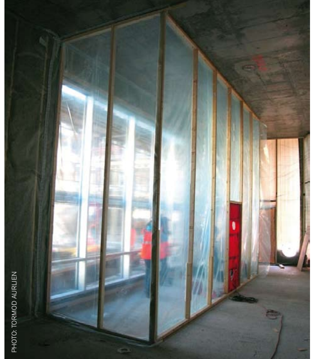
Figure 1. Temporary “tent” made from plastic foil, with a (red) blower door mounted. The amount of air that is sucked out of the tent by the fan in the blower door equals the leaking air that pass through the details of the façade being tested. A person inside the tent may easily detect air-leakages in the façade by just feeling with his hand along joints and details in question, if the air pressure inside the tent is kept at a lower level than the outside (around 50 Pa). This picture is from a new large building with passive-house ambition ( n_{50} < 0.6 \text{ h}^{-1} ).
