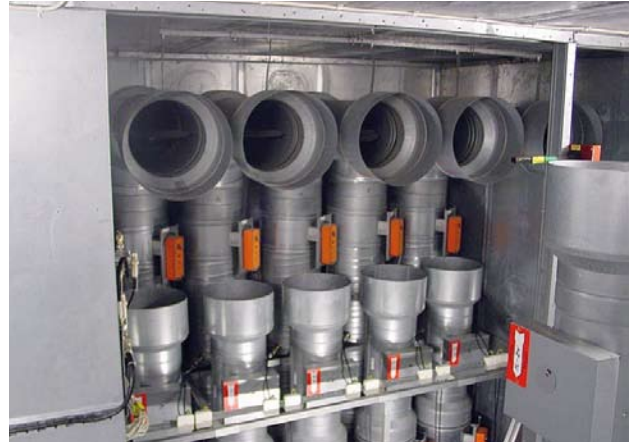
Figure 6. Ducts for the different floors pass down through common shafts, one for supply and one for extract air. The photo shows part of the supply ducts with their fire dampers.
