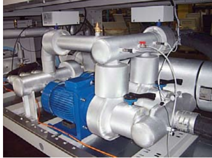
Figure 6. Inverter driven double pump.
