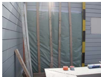
Figure 1. Sealing a large louvre can prove to be a difficult task.
