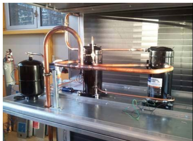
Figure 11. Cooling circuit with tandem compressors in the AHU.
