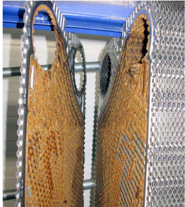
Figure 3. Appearance of the pre-exchanger.
