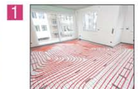
Radiant Heating & Cooling
