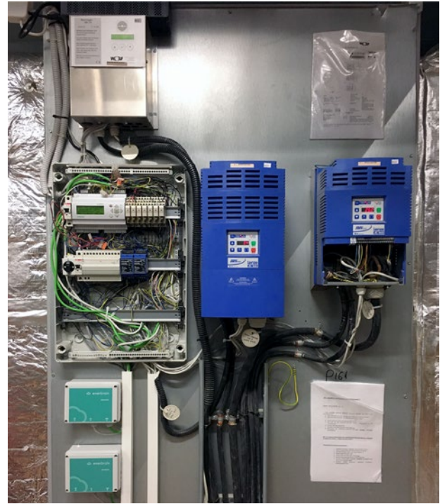
Figure 1. IoT controllers controlling the VFDs of supply and extract fans of AHU 1.
