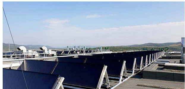
Figure 4. Solar panels installed on the roof.
