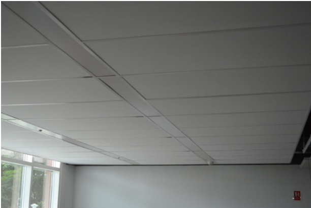
Uponor radiant panel system.
