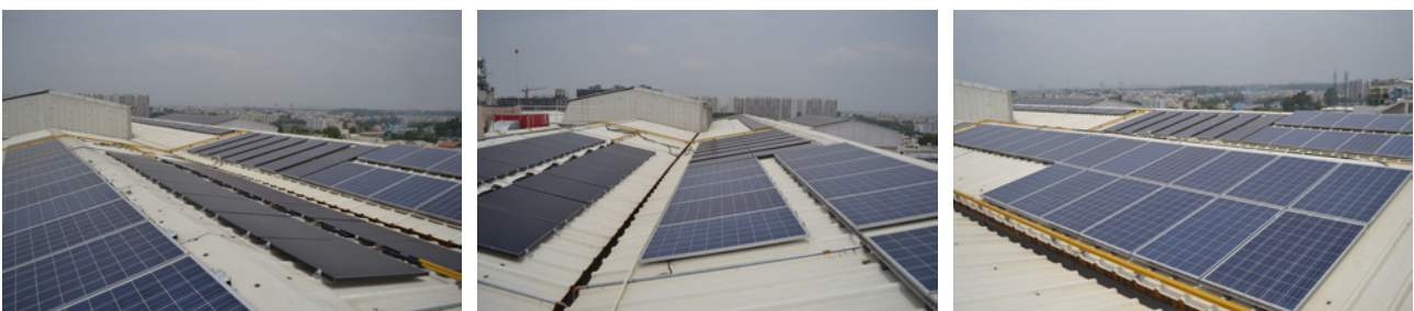
Different solar PV technologies on the roof of EC-53 building.
