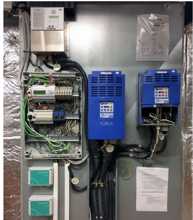
Figure 1. IoT controllers controlling the VFDs of supply and extract fans of AHU 1.
