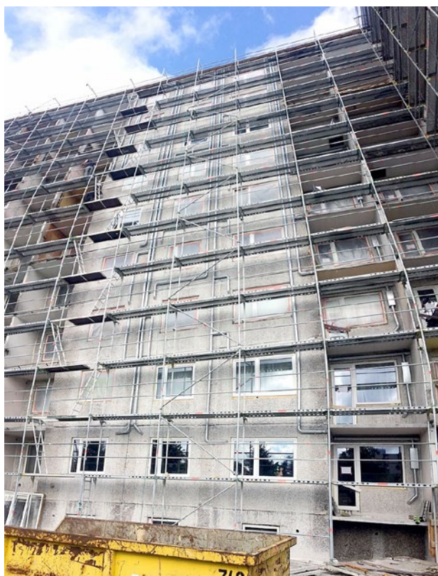
Figure 2. Estonian apartment building renovated with KredEx grant (30% of financial support) that requires to install heat recovery ventilation. On the photo, ventilation supply air ductwork and some parts of extract ductwork are installed on the façade before additional insulation, and heat recovery ventilation unit will be installed to the renovated roof.
