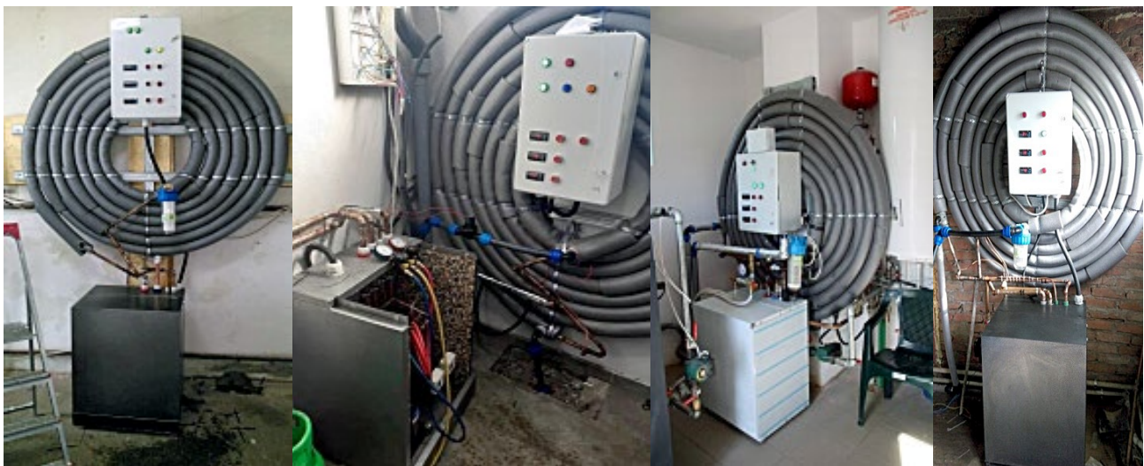
Figure 11. Heat Pumps with Innovative Capillary Evaporators.
