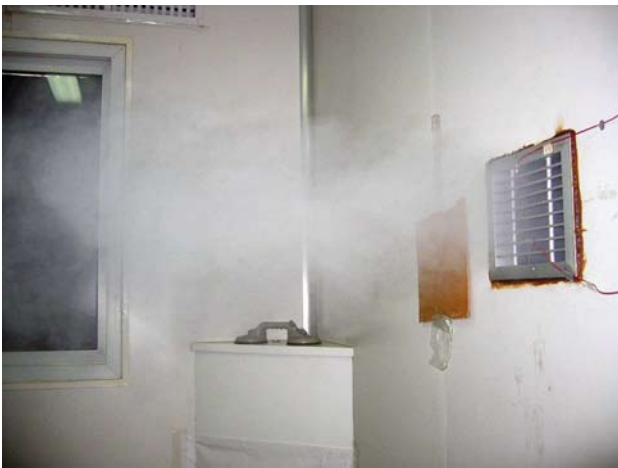
Fig 3. Demonstration of the air supply stratum with smoke.
