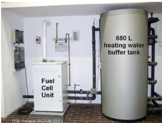
Figure 1. The test arrangement of the BlueGEN natural gas fired fuel cell-based CHP unit manufactured by Ceramic Fuel Cells. Data sheet performance: 0.5–1.5 kW electrical output and 0.3–0.54 kW thermal output. The heating water buffer tank is oversized for test purposes. Laboratory of Heating Technology at Fachhochschule Koeln.
