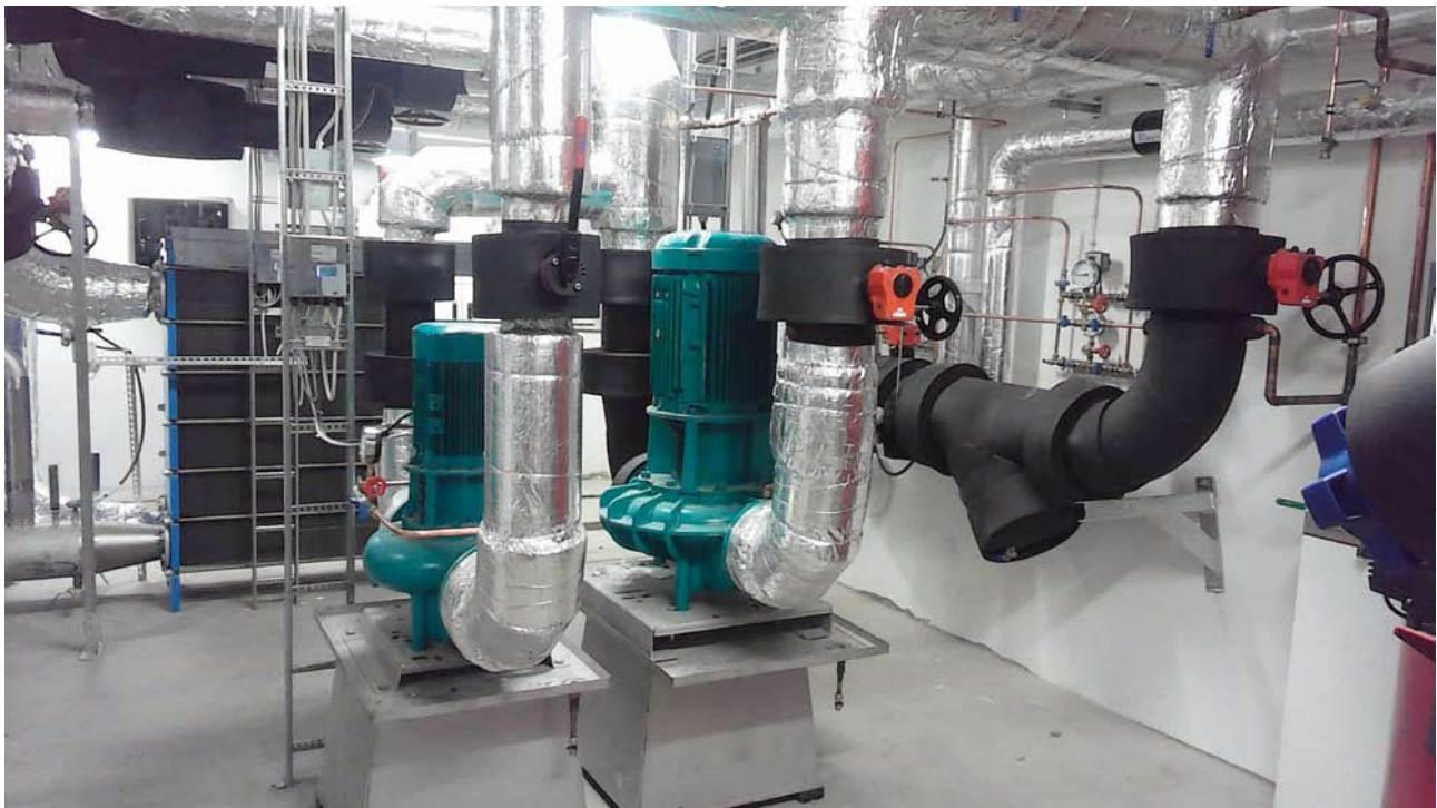
Figure 3. The main circulation pumps for the Skanska Deep Green Cooling in the front and the ground heat exchanger in the rear.
