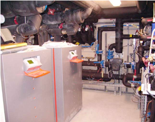
Figure 4. Water/water heat pumps.
