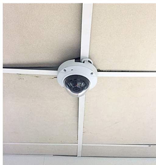
Figure 2. An Installed Camera in the Case Study Building.
