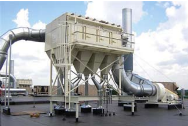
Figure 8. Air Pollution Control (APC) equipment.
