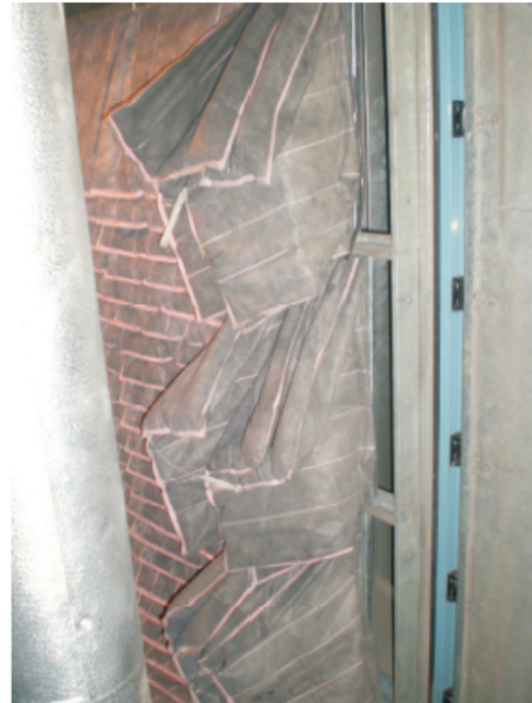
Figure 3. This photo shows two problems. Firstly the gap at the and each row shows an easy route by which the air flow can bypass the filter bank. Secondly nearly all the large sized filters are fitted with the pockets presented horizontally making them choke off the pockets below as gravity pulls them down. Every time two pockets touch there is no air flow through the media in contact. This increases air resistance and energy consumption as a result.
