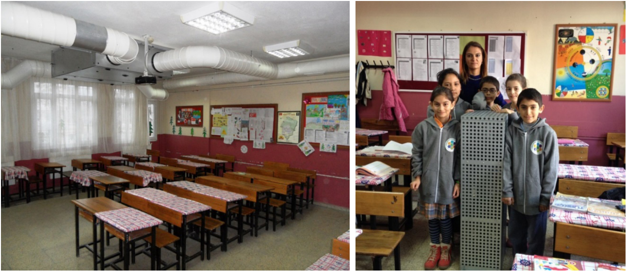
Figure 4. The fitted heat recovery ventilation unit in a classroom and the IAQ team made up of students and the teacher.
