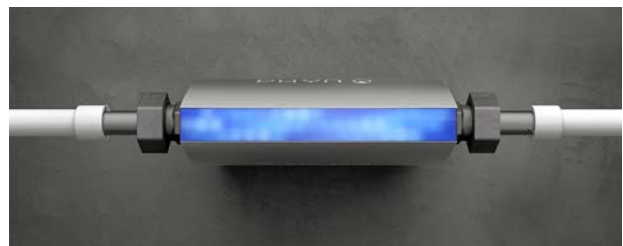
Figure 2. The Phyn Plus unit is installed at the main water inlet of the house and monitors the pressure fingerprints of each consumption point from this single location.
