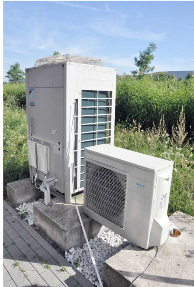
Figure 2. Daikin Altherma outdoor unit (right) and VRV outdoor unit (left).
