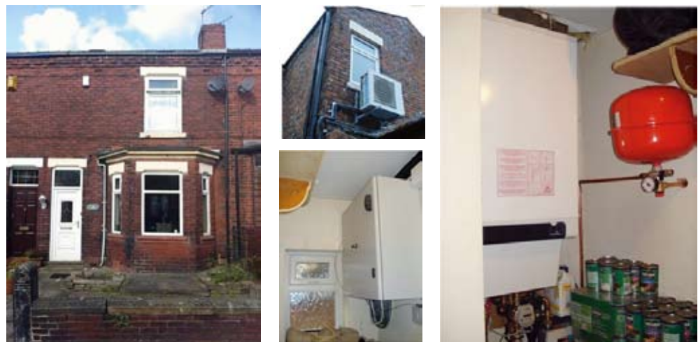
Figure 4. The HYBRID heat-pump system was tested in this 110 year old, terraced UK house during winter 2011-12. A family of three lived in the building with heated floor area of 140 m 2 . The house was heated with hot water radiator system with design supply temperature of water 70°C in design outdoor temperature of -6°C.
